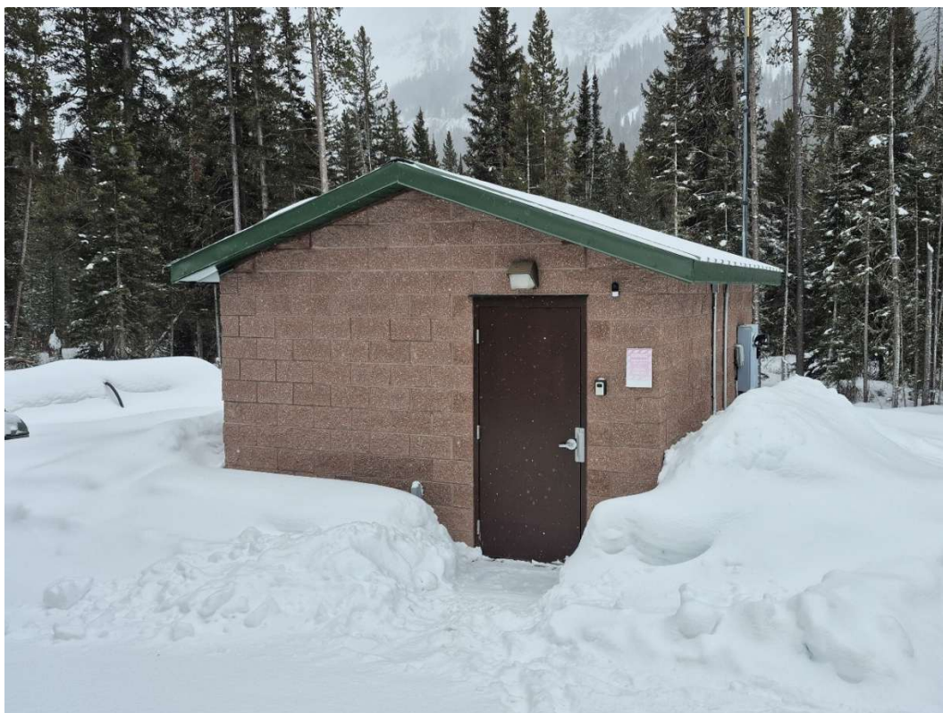
Figure 2 -Pump House (Exterior)
