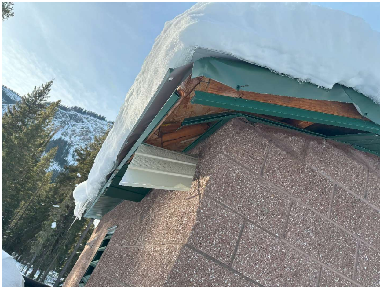
Figure 8 – Failing Well House Roof
